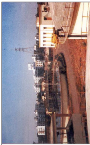
CHINCHWAD SEWAGE TREATMENT PLANT
